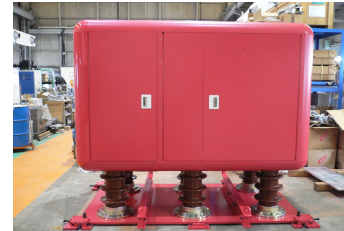
Figure 10: Photograph of the high voltage terminal box
