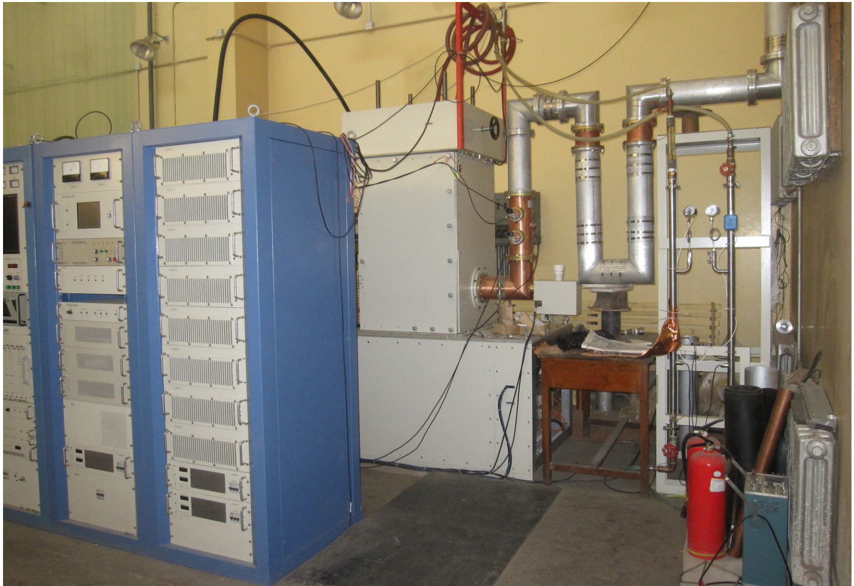
The power generator and transmission line installed with test cavity.
