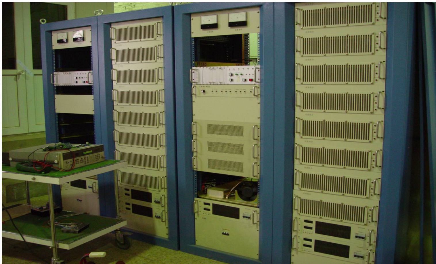
The 6kW driving power amplifier and monitoring devices
