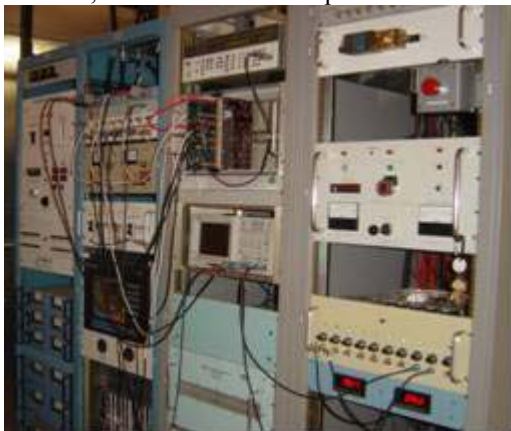
Figure 5: LENS klystron RF transmitter racks.
