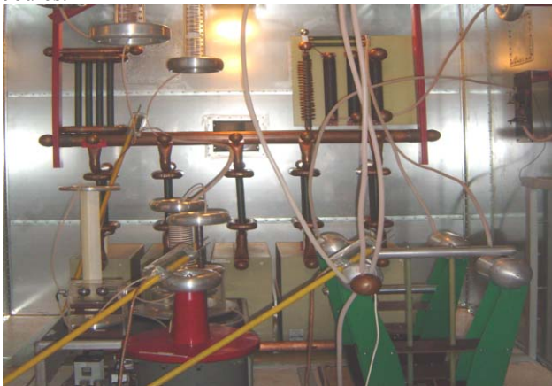
Figure 4: HV capacitor bank with plastic capacitors.
