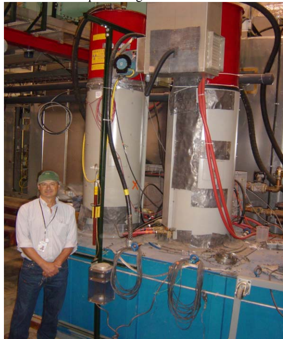
Figure 6: LENS klystrons and modulator tank.
