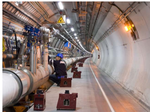
Picture 3: LHC 27 km Liquid He transfer lines
