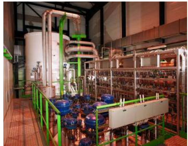
Picture 1: A LHC 18 kW cold box
