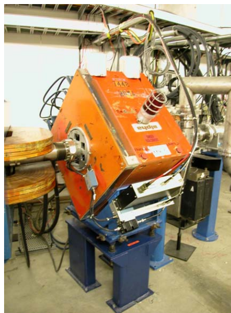
Figure 2: ECD Installed in PSR quadrupole.
