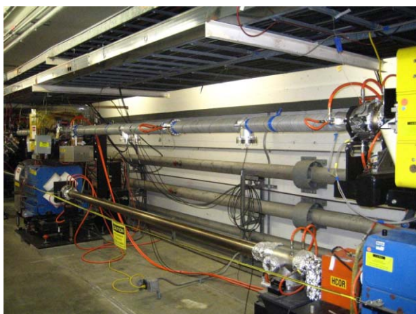
Figure 2: Detail of the LER vacuum chamber in IR12 (upper beam pipe). The inner clearing solenoid can be seen.
