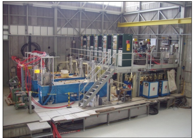
Figure 2: MTE kicker generators.
