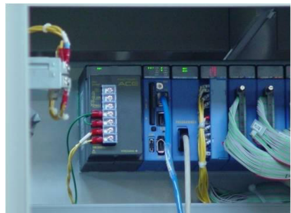
Figure 2: F3RP61 in operation.
