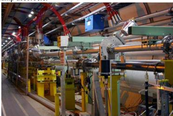
Figure 3: LSS picture showing the dump line installed on top of the circulating beam pipe.
