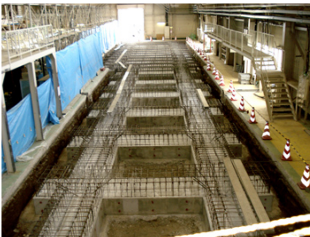
Figure 5: ATF2 floor construction : A 0.6m thick concrete slab of 396m 3 will be supported by 0.6m thick beams, which are visible in this picture, and 38 piles with 0.7m diameter and 13m height, which were buried under the beams.
