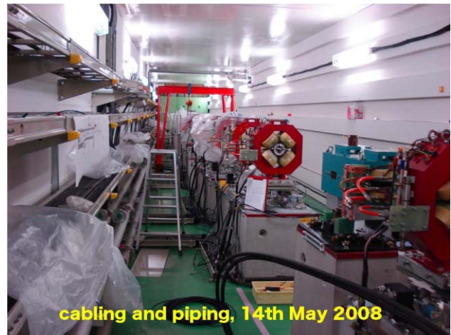
Figure 6: ATF2 beam line under construction : all the quadrupoles and bends were installed with cable and cooling pipes.
