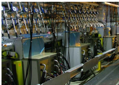
Figure 2: Kickers and amplifiers in the LHC tunnel.
