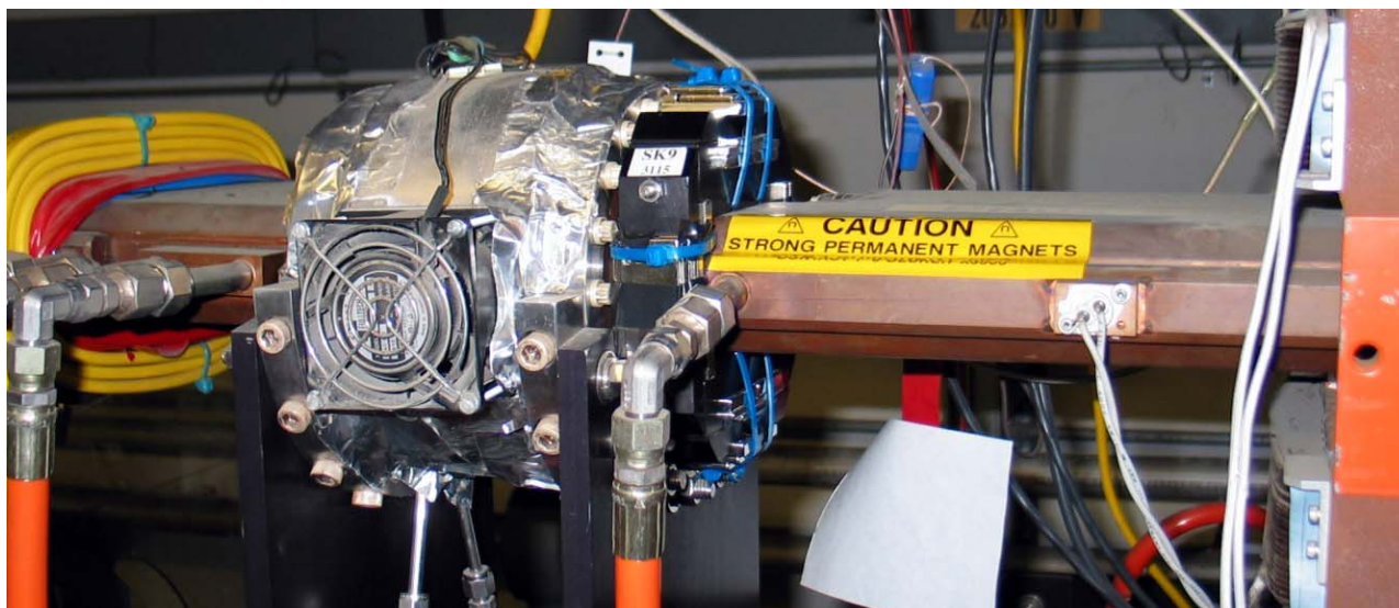
Figure 3: Permanent magnet skew quadrupole (SK9) installed on the beam line. The space for these magnets is very restricted, there is about a 1.5 to 2 inch gap in the cooling channel on the side just after a bellow (with fan here). Solenoid windings (yellow, left) to suppress electron cloud were sometimes in the way and had to be cut by a few windings. The iron of the quadrupoles or correctors (orange, right) should be far enough not to influence the field. The only magnetic metal near the skew quadrupole is the water pipe fitting at the orange hose (middle).
