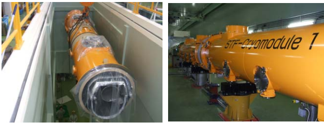
(a) Transfer to underground tunnel (b) Completed Cryomodule Figure 4 Final assembly of STF Cryomodule
