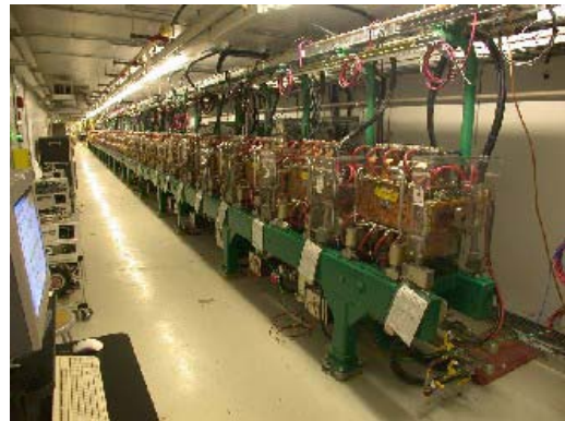
Figure 5: CCL in the tunnel.
