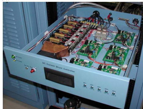
Figure 1: View of a chassis containing 5 shunt circuits
