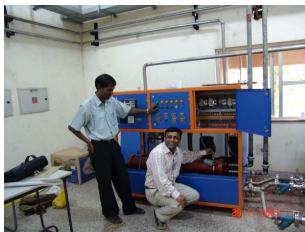
Figure 4: 5-Ton Chiller Unit and its Control System
