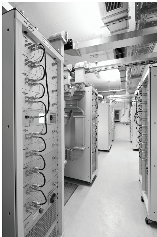
Figure 1: The RF power amplifier gallery of ELBE.
