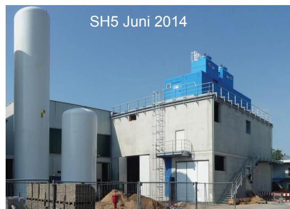
Figure 5: The new hall SH5 for the cryoplant that serves the SIS100 magnet series test facility. The installation work will be completed in August 2014.
