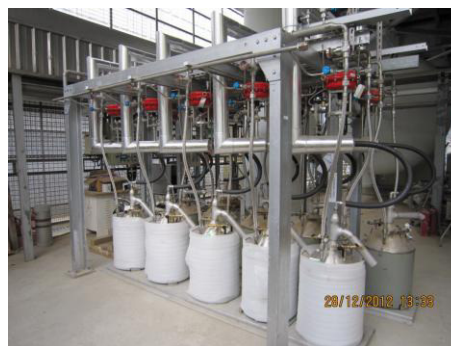
Figure 3: Two arrays of purifiers cooled with liquid nitrogen.
