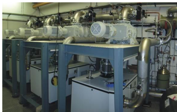
Figure 2: Four parallel switched Pumping Units.
