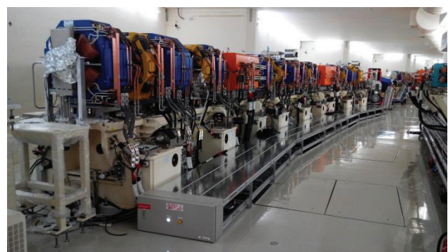
Figure 6: TPS SR installation status.
