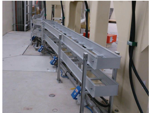
Figure 9: TPS LTB cable tray.
