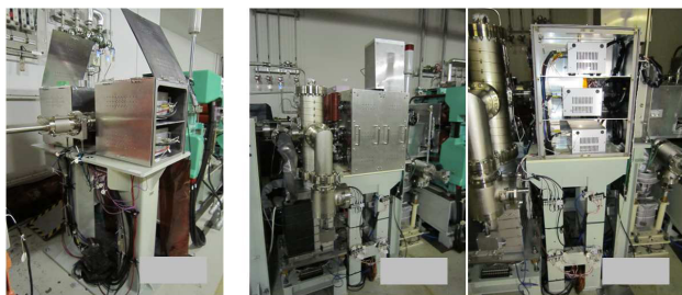
Figure 1: Installed fast correction kickers in the SPring-8 storage ring. Left photo shows the primary fast correction kicker system. Right photo shows the secondary one. The power supplies driving the kicker are put in the radiation and noise shield boxes on both side of the kicker.
