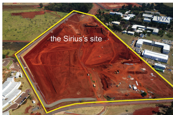
Figure 1: The future site for Sirius and the old light source UVX (on the top right side). The earthwork is already concluded and construction should start soon.
