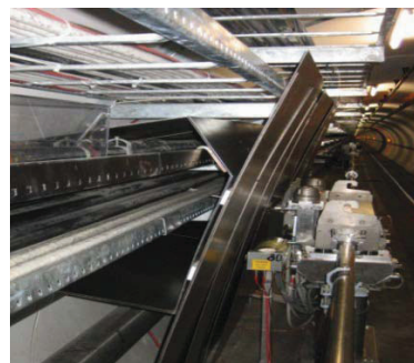
Figure 6: Magnetic shielding installed on the collimator TCDIH.29050 on May 2009.
