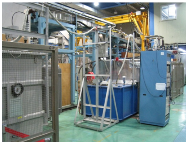
Figure 3: Installed modulator at KAERI.
