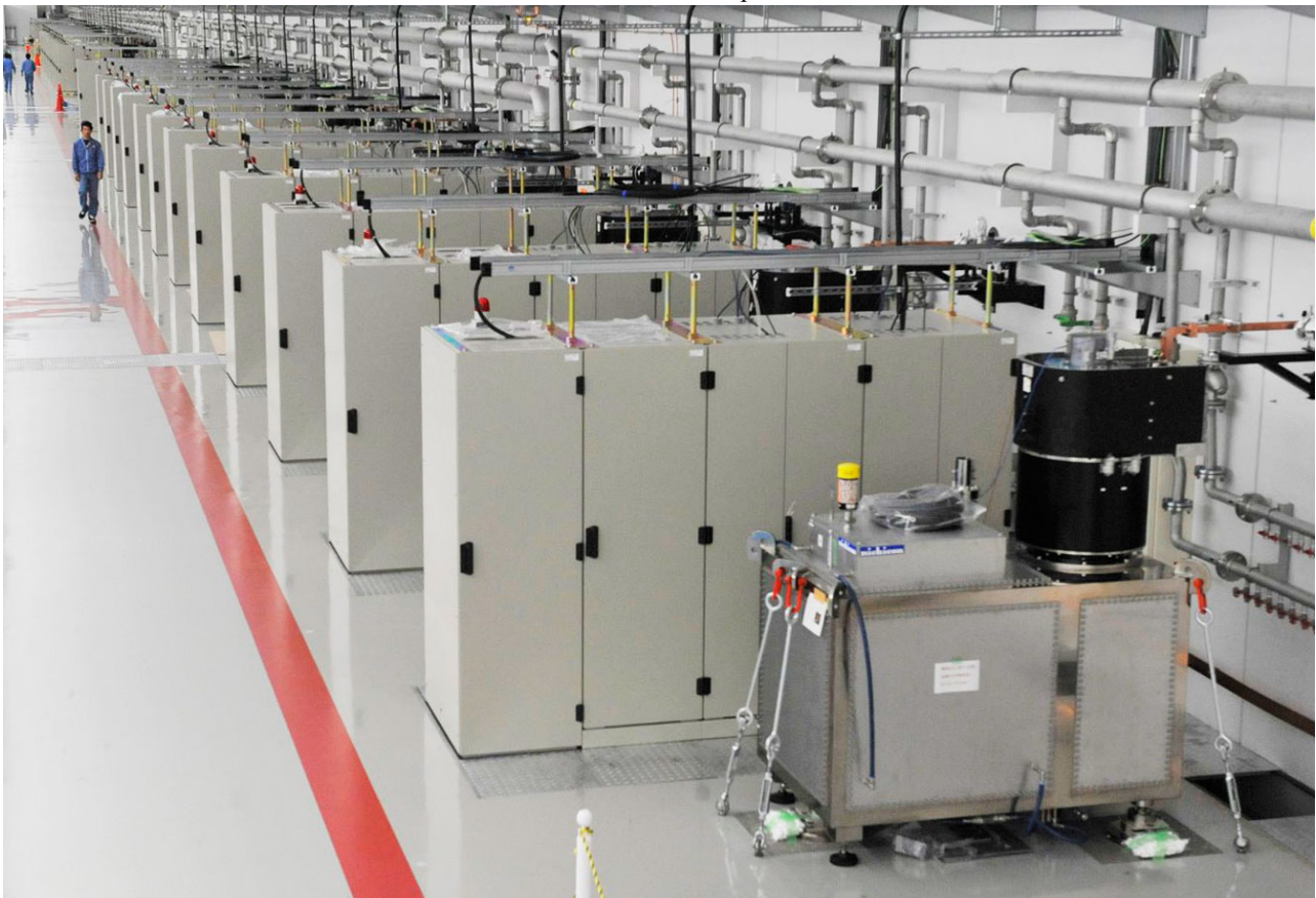
Fig. 1 Installed single-tank compact klystron modulators. In each 4 m section, we install C-band klystron modulators and control cabinets, which house the VME control, low-level rf system, inverter HV charger and vacuum controls.
