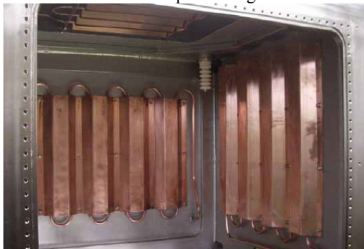
Water cooling pipes mounted on window panels.
