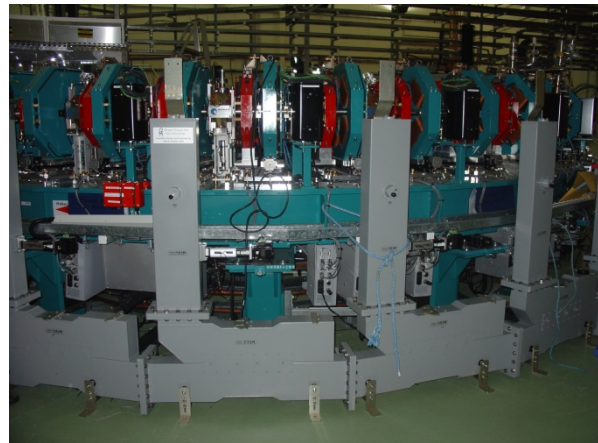
Figure 5: RF Waveguide Distribution System Installation.
