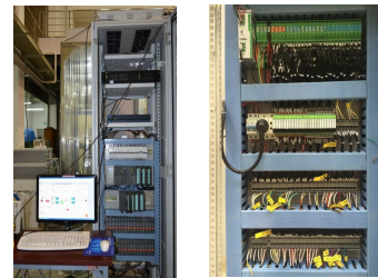
Fig. 4 Left: The ion sources control system based on PLC of Siemens S7 series 300.
