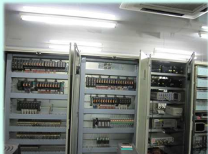
Local Control Cabinet
