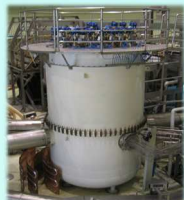
Distribution Valve Box
