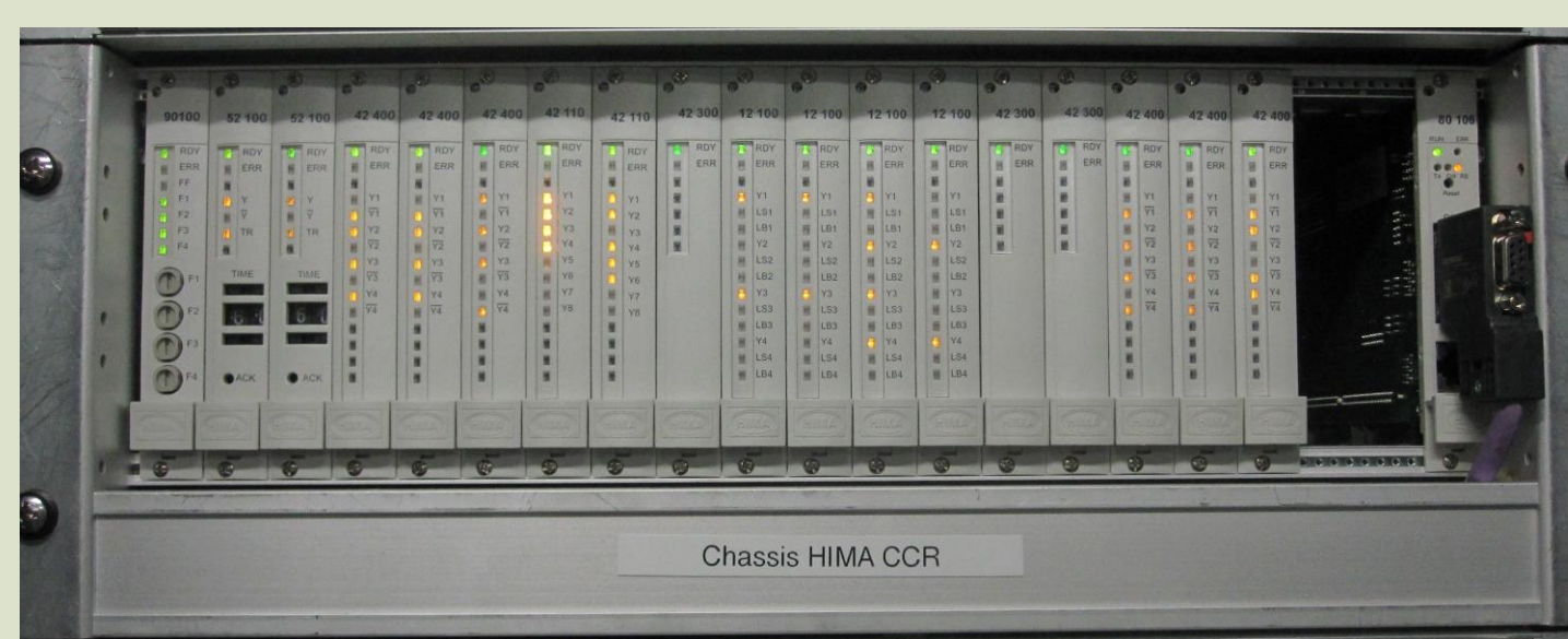
HIMA Planar4 wired logic in a 19-inch sub-rack of the SPS primary ion interlock. From the left: fuse module, two timing modules, logic modules, and far right a Profibus supervision module.
