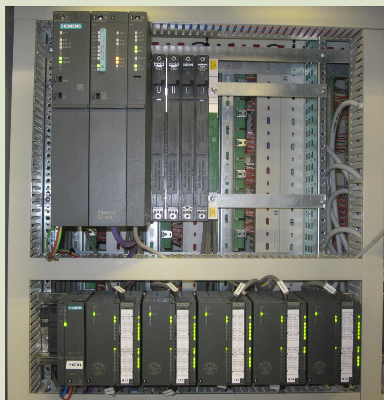
Siemens S7 400 CPU and ET200 remote I/O modules of the PASS key controller.
