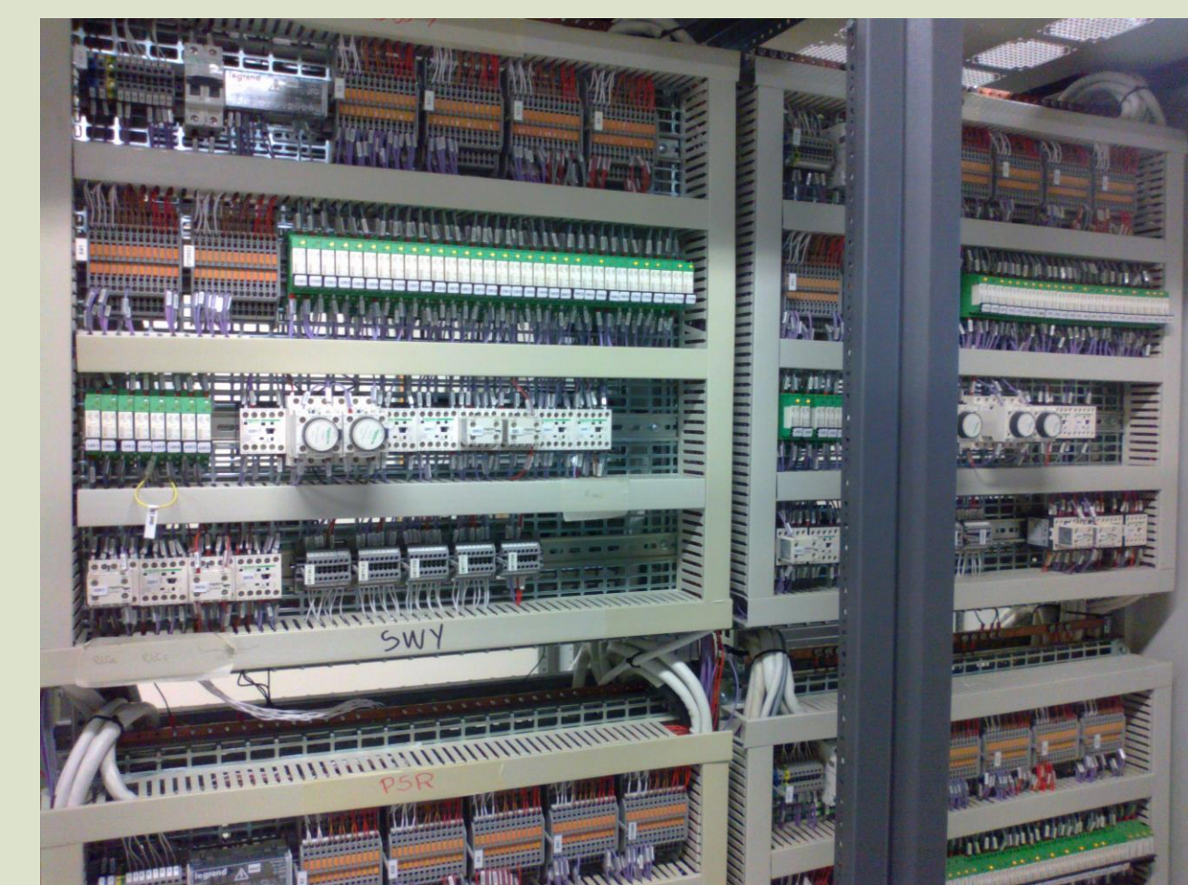
Hardwired relay-based wired logic of the PASS cabled loop. Green LEDs indicate contact states.
