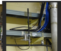
FIG. 7: Photograph of collinear antenna for Wireless LAN in the linac tunnel. 10
