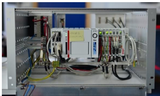
Figure 4: One of the main ESPRESSO PLC CPUs placed in a 19" sub-rack.
