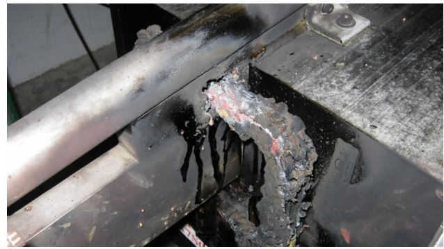
Figure 1: Septa magnet MYR7S03 fire damage.
