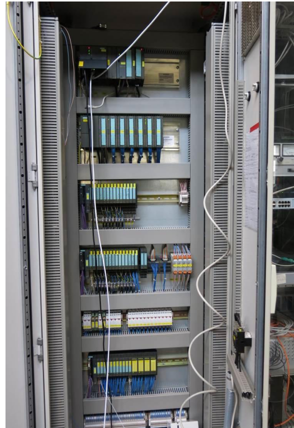
Figure 4: Main cabinet with PLC and 3 ET200S systems.
