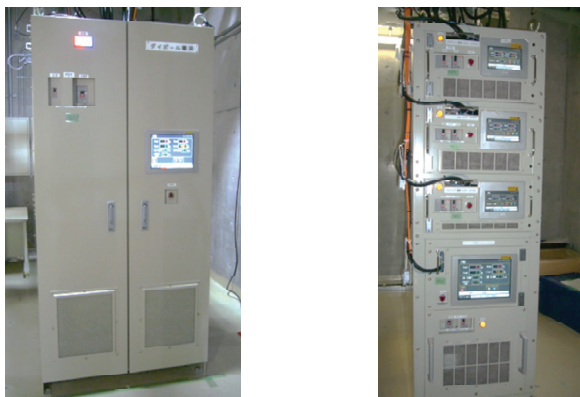
Figure 3: Pictures of the new power supplies for the normal-conducting magnets. The left photo shows a power supply for a dipole magnet and the right shows four steering magnet power supplies installed in a rack.
