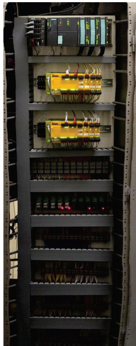
Figure 2: New Installation in repurposed racks.
