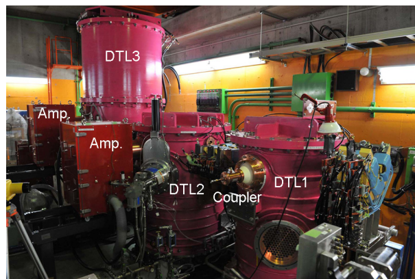
Figure 5: Photograph of DTL resonators of RILAC2 placed in AVF cyclotron room.
